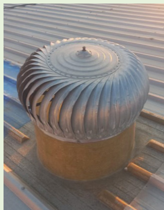
Wind ventilator and turbojet fans are installed in the Sohna plant to improve shopfloor ventilation.
