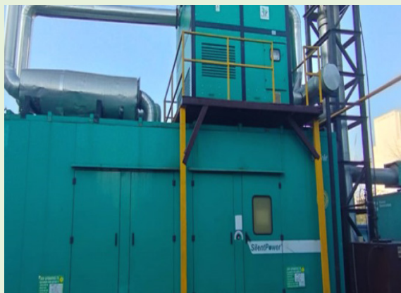
Retrofit Emission Control Device (RFECD) is installed at IMT I & Sohna plants to reduce emissions.
